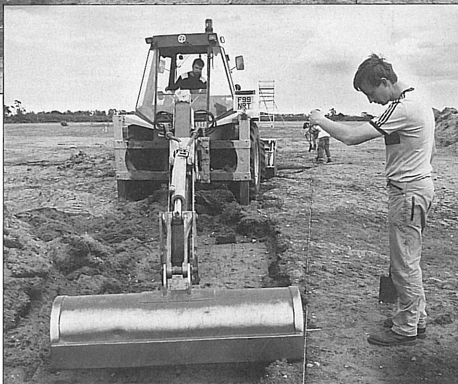
Top: Opening up Sector 1 by machine at the start of the 1990 season. Bottom: Andrew Copp supervises the machine driver.
