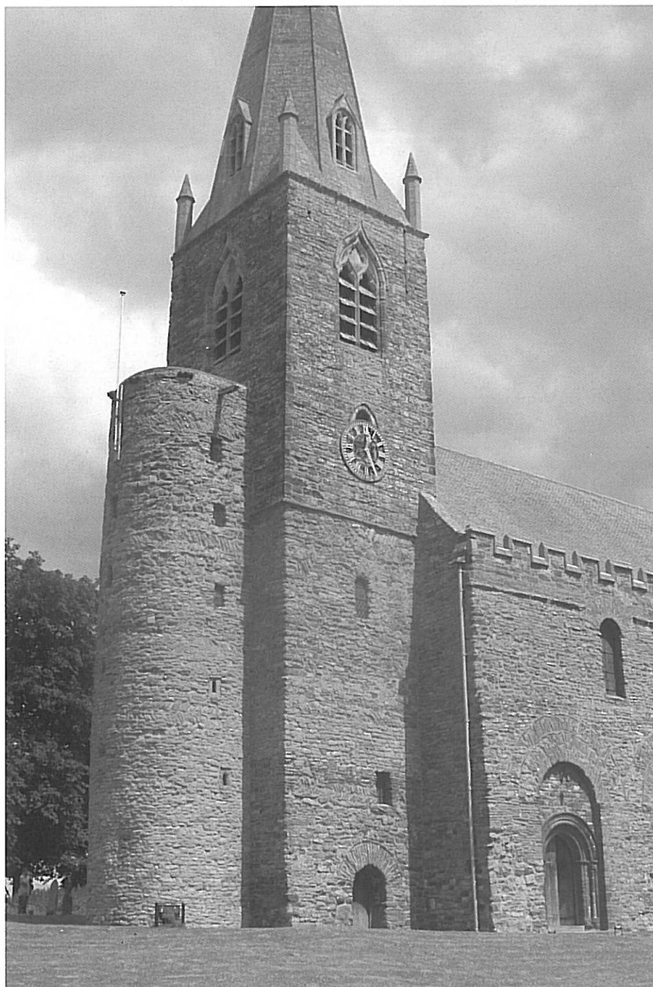
Brixworth Church with 11th-century round stair turret. The stone spire is 15th-century
